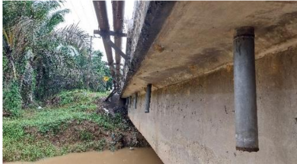
Gambar 2. 12 Pipa drainase jembatan
